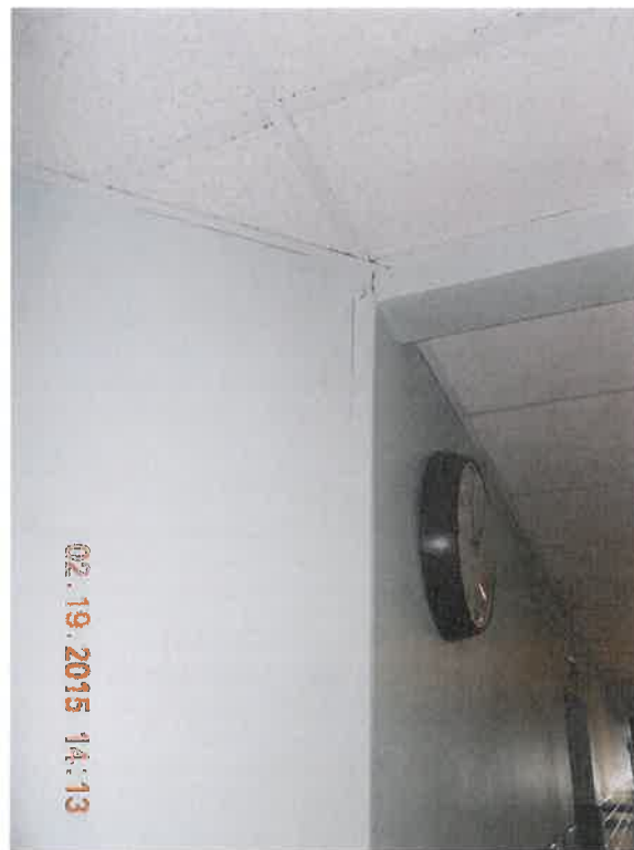
Cracks caused by absence of deflection track
