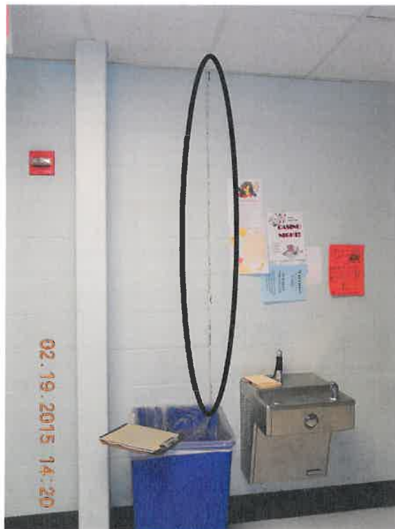
3rd floor corridor - failed control joint due to inadequate thickness of caulking.
