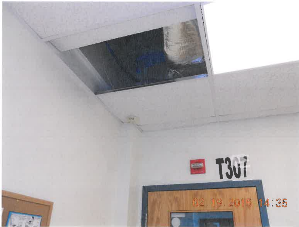
Water damage above ceiling.
